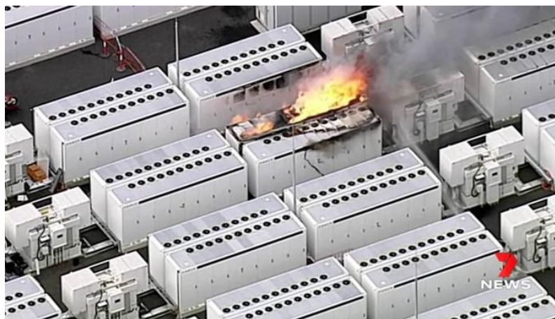
Rys. 7 Pożar magazynu BESS Victoria Tesla Big Battery 300MW/450MWh Source : https://reneweconomy.com.au
